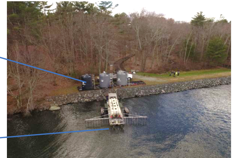
Staging area, chemical storage tanks, and treatment vessel on April 26, 2018.
