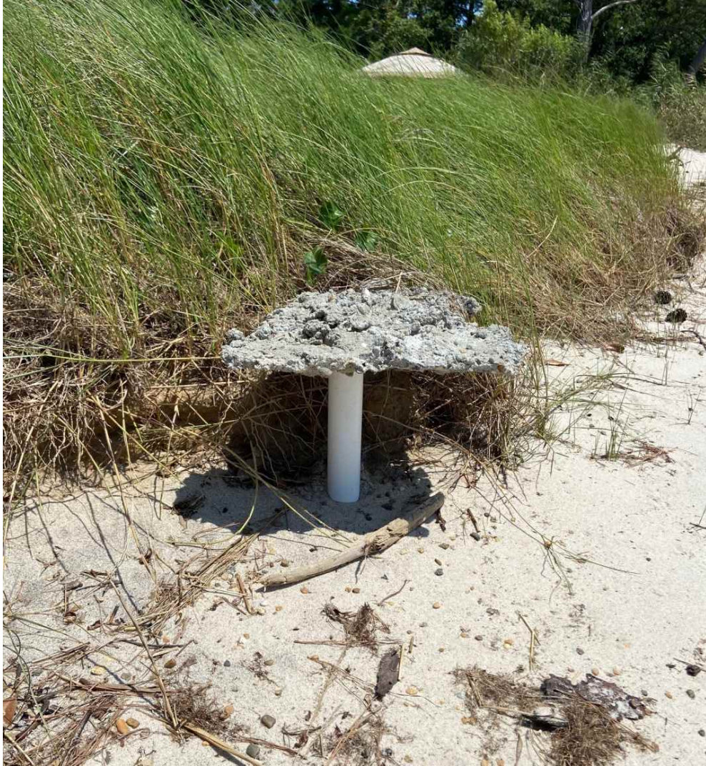
Incorrectly abandoned monitoring well
