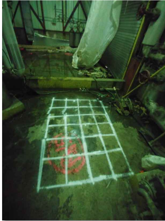
Rebar identified during GPR scanning
