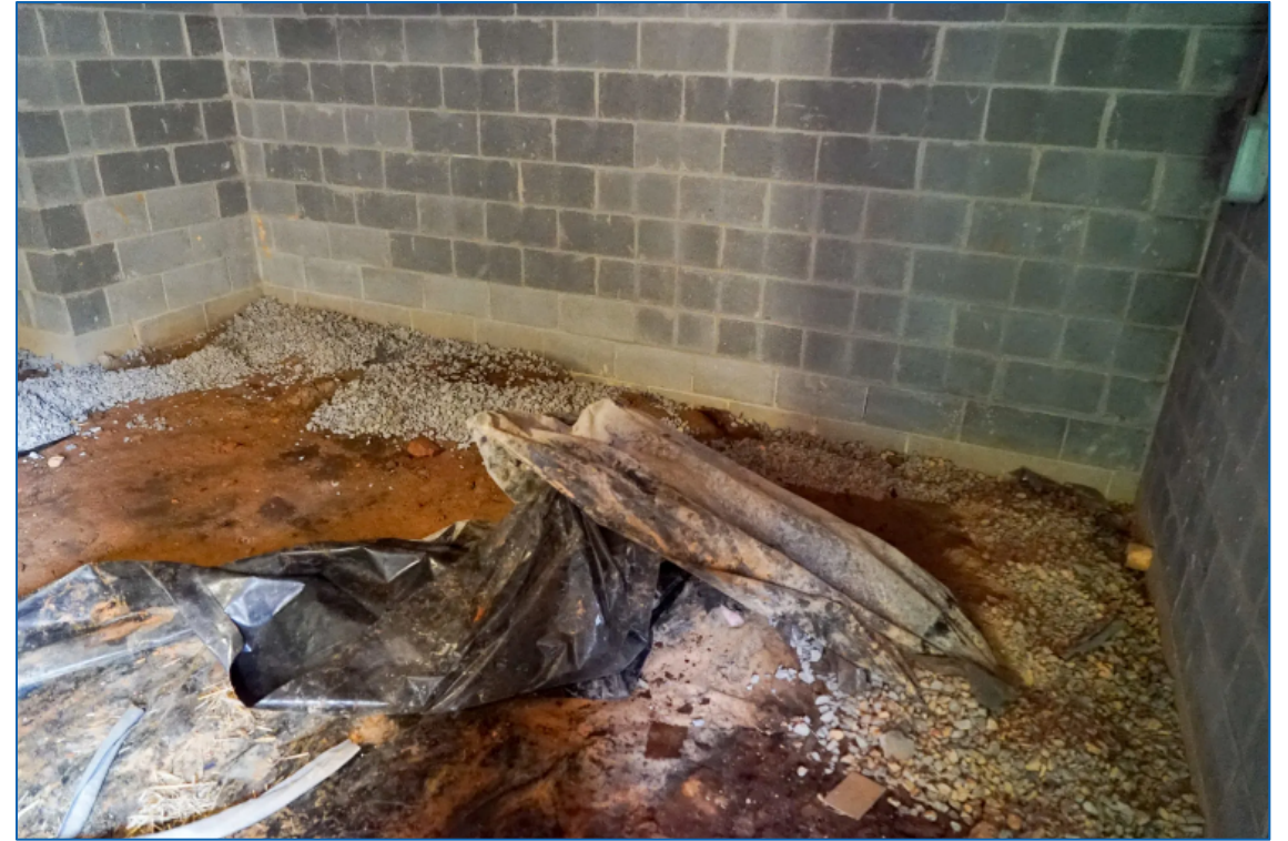
Damaged vapor barrier by third party contractors
