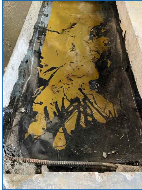
Damaged barrier with rebar
