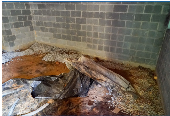
Damaged vapor barrier
