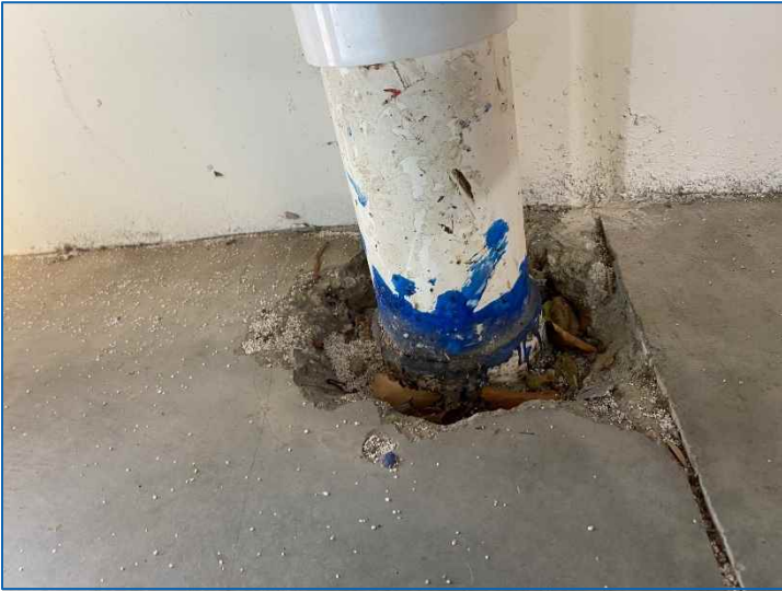
Damaged concrete above barrier
