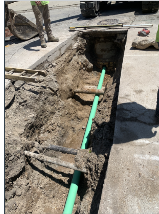
1 Manhole Extraction Point (trenched)
