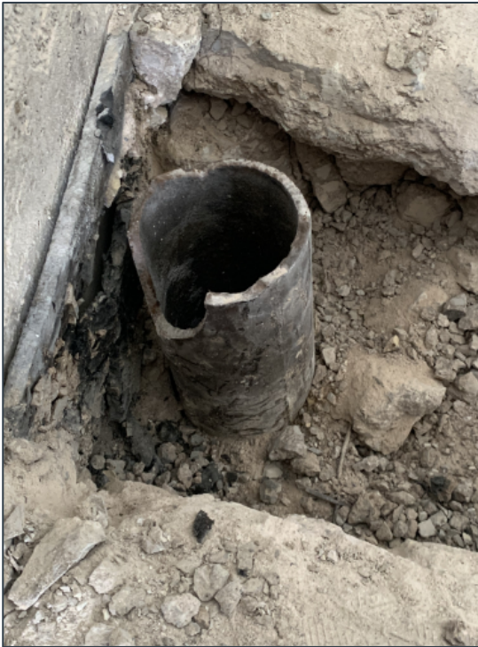
2 Sewer Cleanout Extraction Points
