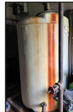
AFFF storage tank
