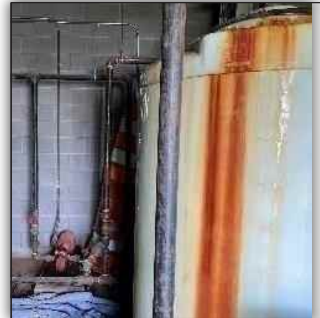
AFFF storage tank
