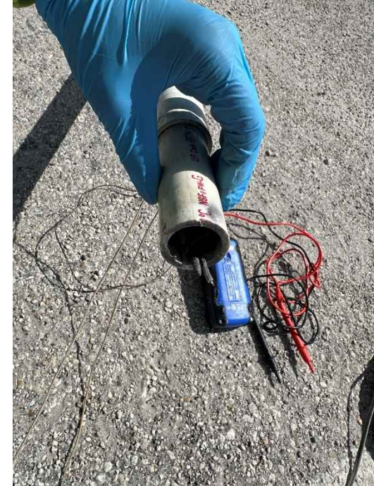
Broken connection between anode and cathode.
