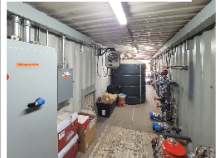
Full-Scale Dosing System
