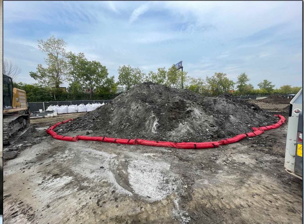
Lead Contaminated Soil
