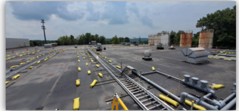
Rooftop Cable Trays and Piping Runs
