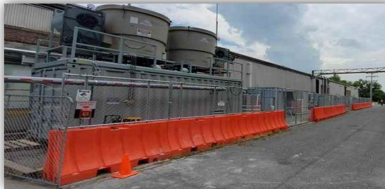
Exterior ISTR Treatment System Equipment
