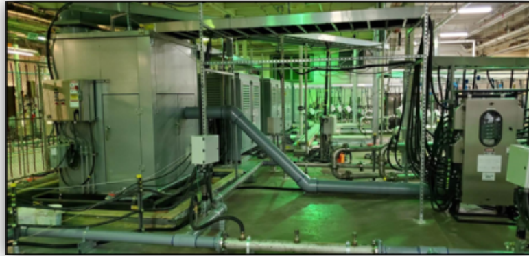
Interior TCH System Process Equipment
