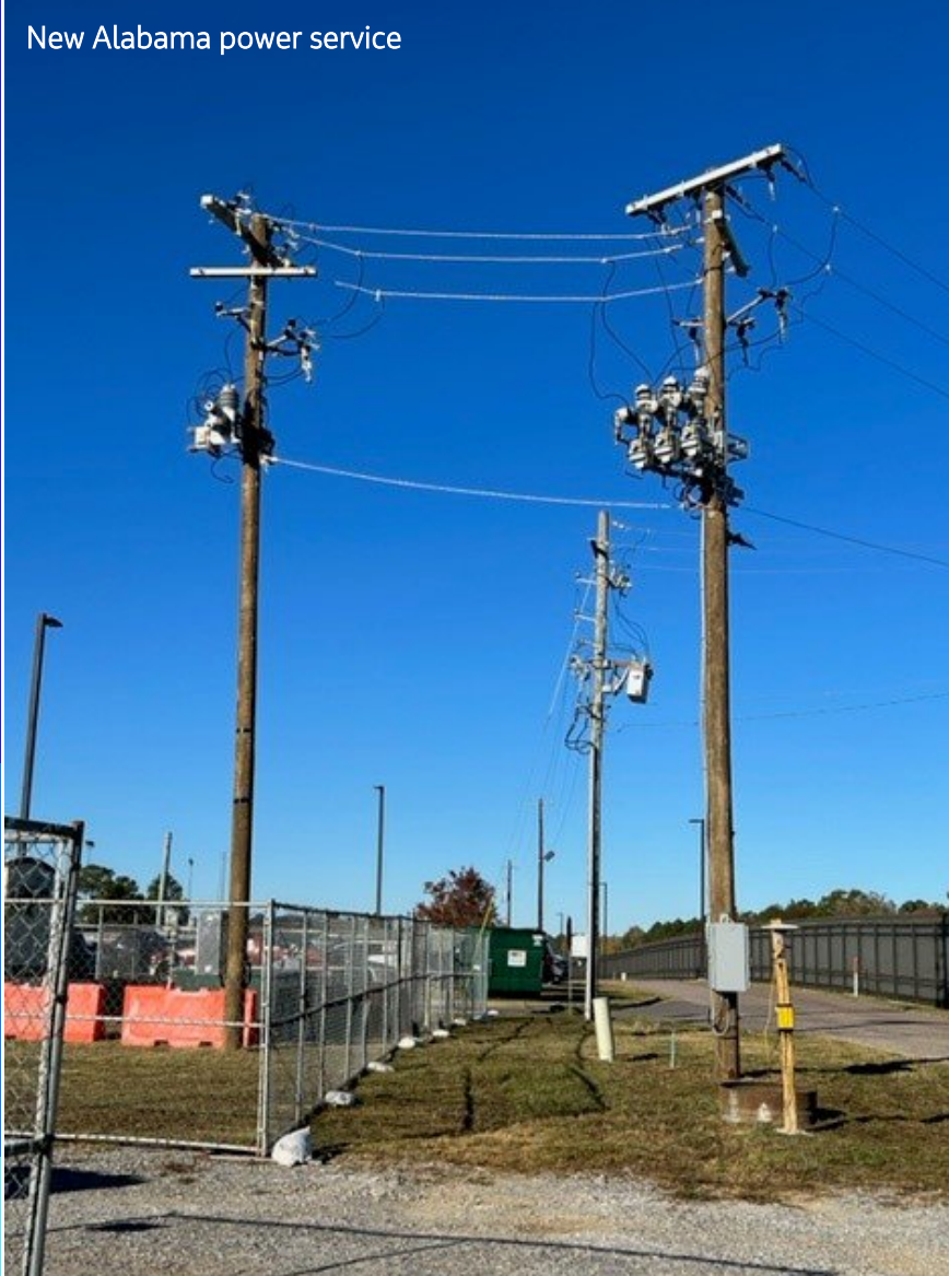
PCU and output power cables
