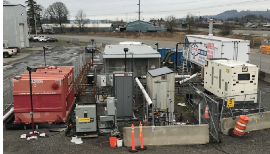
Steam Boiler and Extraction and Treatment Equipment
