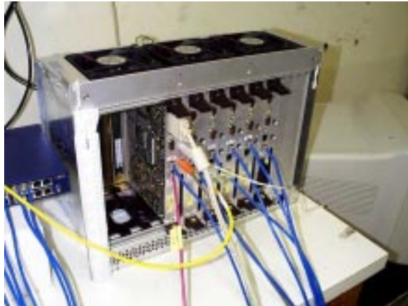
Figure 1. Air Management Node "Cage" ¾ View
